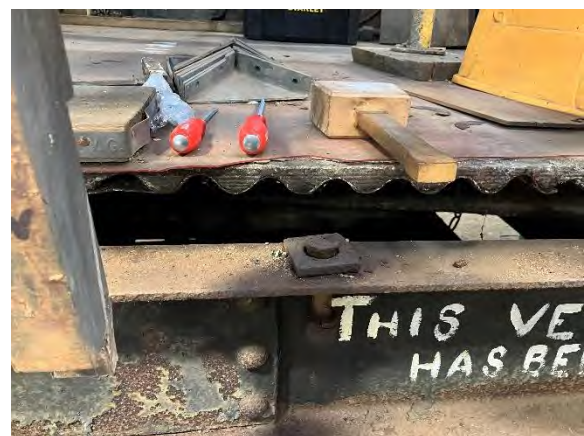
The SW corner of 7864 stripped down, with work proceeding to remove the top lights (top). The lower half of the bodyside framing, showing the rotten residual bottom side (middle). The area on the right once the rotten timber had been cleared out (bottom). March 2024. Photos: Keith Leppard
