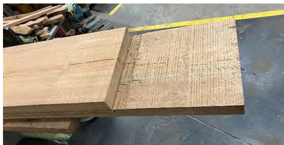
The SW corner pillar under repair, using hardwood plugs to fill cored-out holes where steelwork has been removed (top), and the first new bottom side lap joint before fettling (bottom), March 2024. Photos: Keith Leppard
